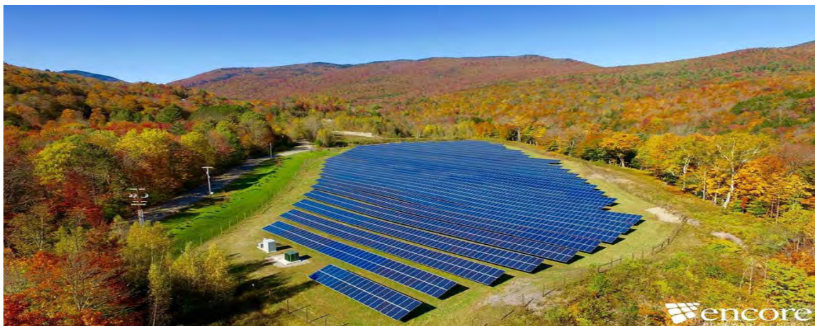
Figure 89: Stowe's Nebraska Valley Solar Farm (1MWAC)
